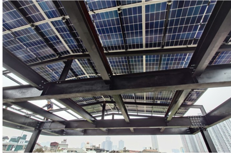
Figure 2. The rooftop grid-connected solar power system using bifacial PV
