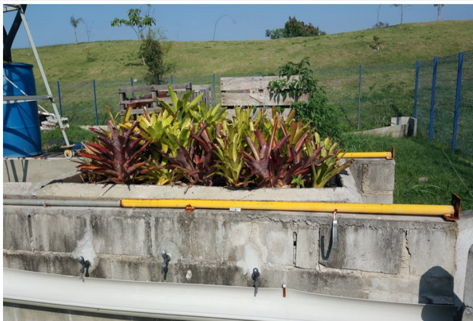
Figure 11 - Green roof and the drains
