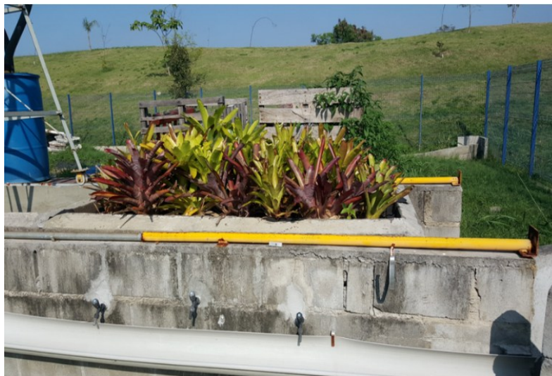
Figure 11. Green roof and the drains
