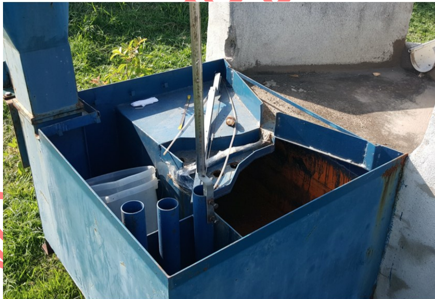
Figure 6 - Rain Gauge Box and the Level Meter [52]
