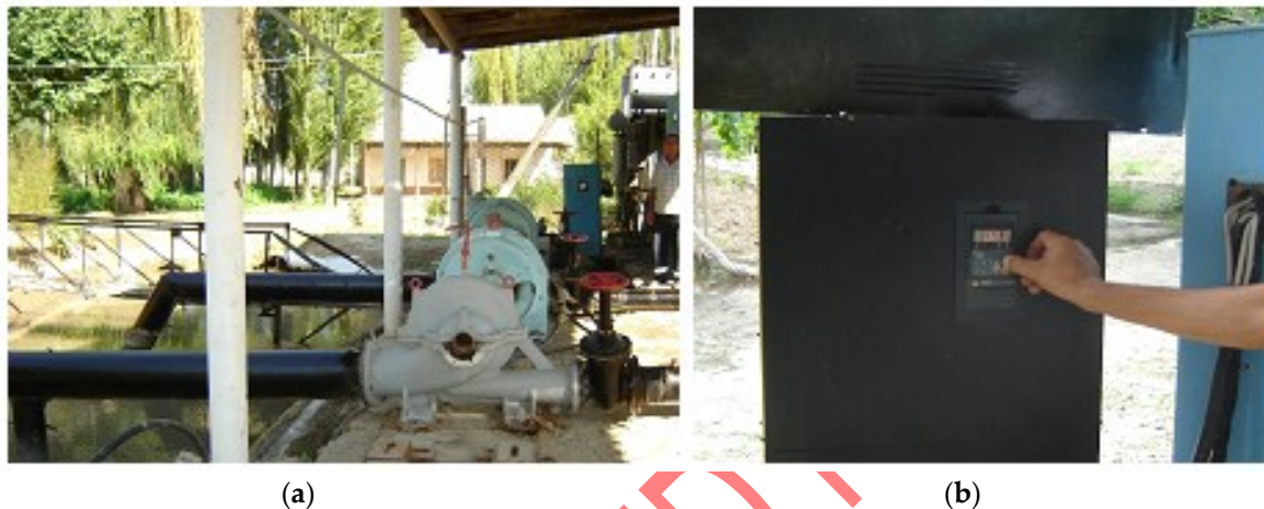
Figure 4. Pumps 200D-90 (a) and frequency and frequency converter (b) at Teshiktosh-1 irrigation pumping station
