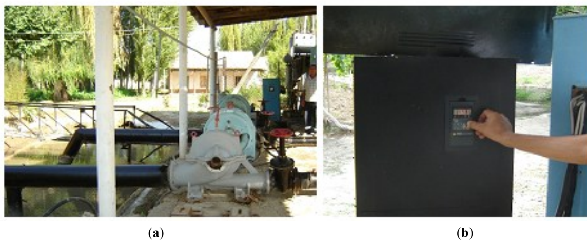
Figure 4. Pumps 200D-90 (a) and frequency converter (b) at Teshiktosh-1 irrigation pumping station
