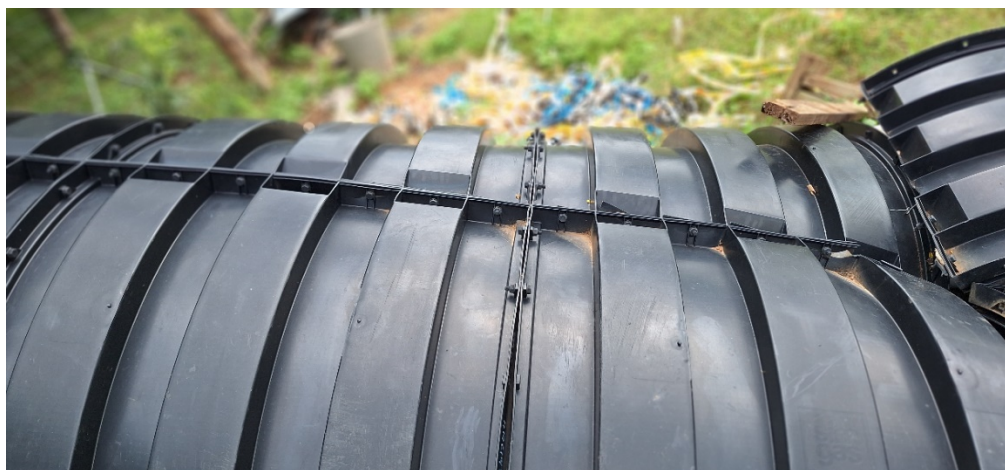
Figure 1. A plastic biogas dome material that was assembled onsite but has to be replaced soon because of poor workmanship and deterioration of the material due to exposure to sun
