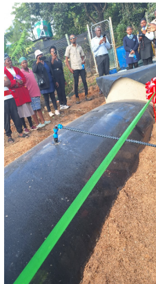
Figure 3. Inflatable fixed biogas dome recently constructed by STREEC and inaugurated by the Eswatini Mistry of Natural Resources and Energy
