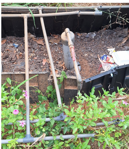
Figure 2. A plastic biogas dome installed underground but no longer functional due to lack of feed material and water
