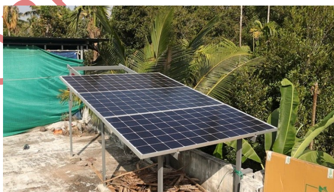
Figure 3. Solar panel setup
